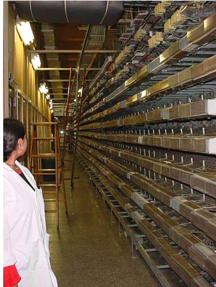
MDF: Main Frame Distribution
